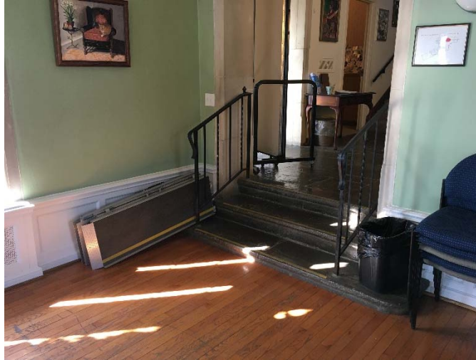
Portable ramps are used as means of accessibility to a major main level space.
