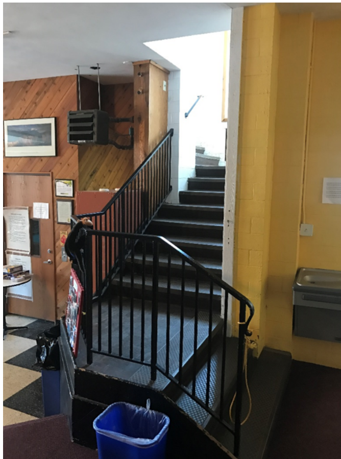
Main level stairs; multiple levels present accessibility challenges.
