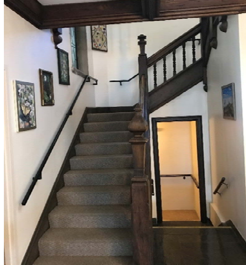
Multiple level changes, narrow doorways, and non-code compliant stair and railings are found throughout the existing facility.
